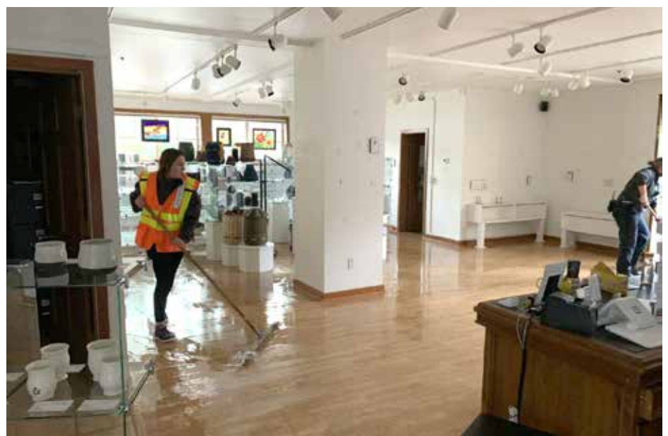
A worker clears two inches of water after a hard freeze broke water pipes on the 3rd floor. Photo by Nancy Frances
